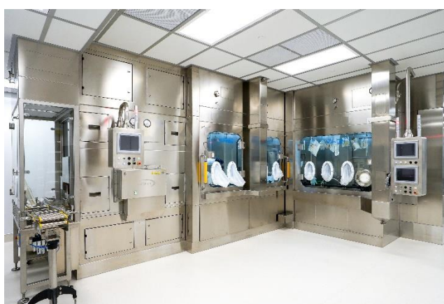
Fig. 2 – The line for processing glassware in RTU tubs
